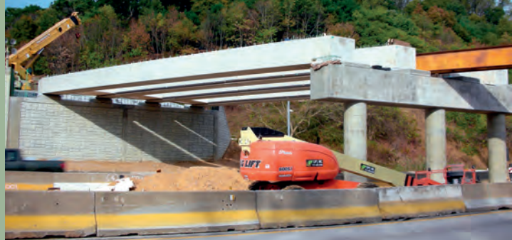
ABOVE: Crews set the beams on the Mill Road bridge over Route 202.
